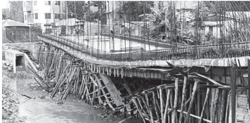
Even after a year, the bridge over Louhajang river in west Tangail is in its worst shape due to the delay in the reconstruction works. Earlier, the bridge collapsed after half its construction was completed.
