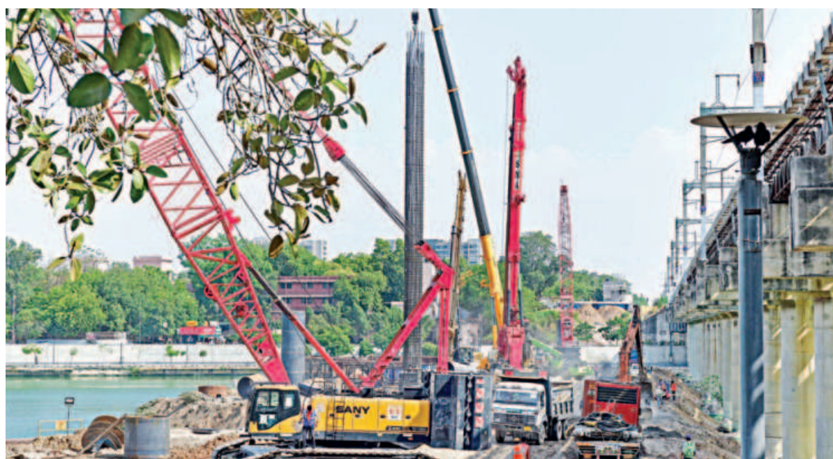
Heavy machineries are seen installed at the construction site of the Mumbai-Ahmedabad high-speed rail corridor across Sabarmati river in Ahmedabad on May 18. PHOTO: AFP
