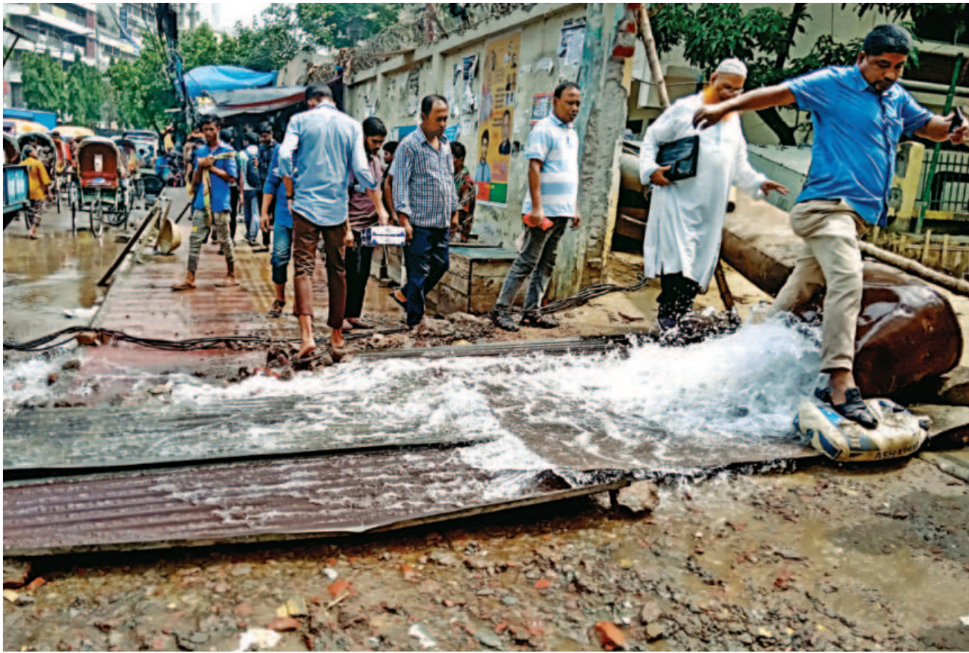
Water from Fakirapool Wasa pump station being drained over the pavement as a new water pump is being installed there yesterday. The authorities apparently had no regard for the difficulties they were putting pedestrians into. PHOTO: ANISUR RAHMAN
