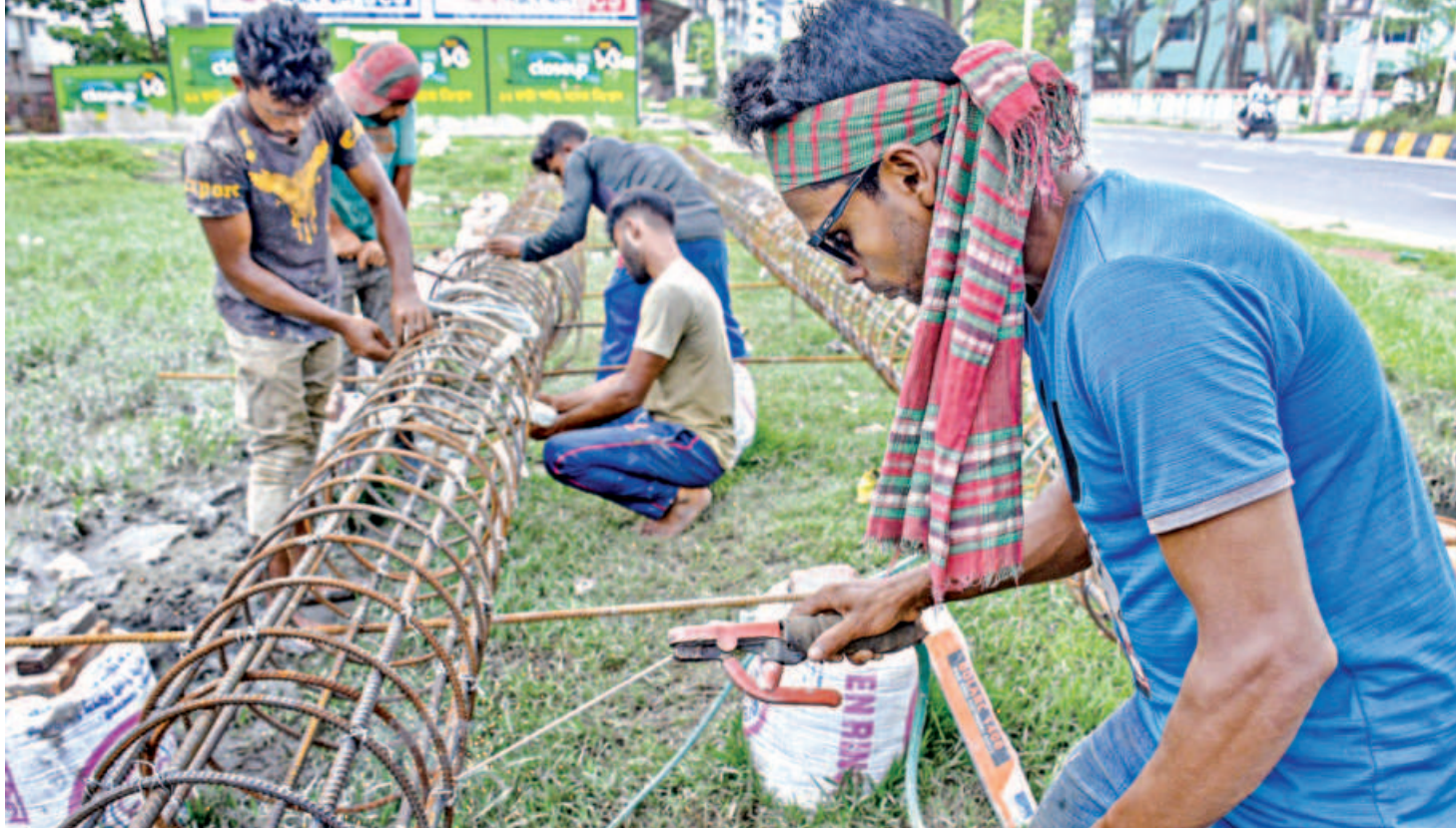
Workers build cages bending and welding together steel rods for piling foundations into the ground. The piles are built under different structures to transfer loads from the structures to the ground, helping to support them. Five workers can prepare anywhere from five to six cages in a day, earning Tk 600 each. The photo was taken from Khulna city on Sunday.
