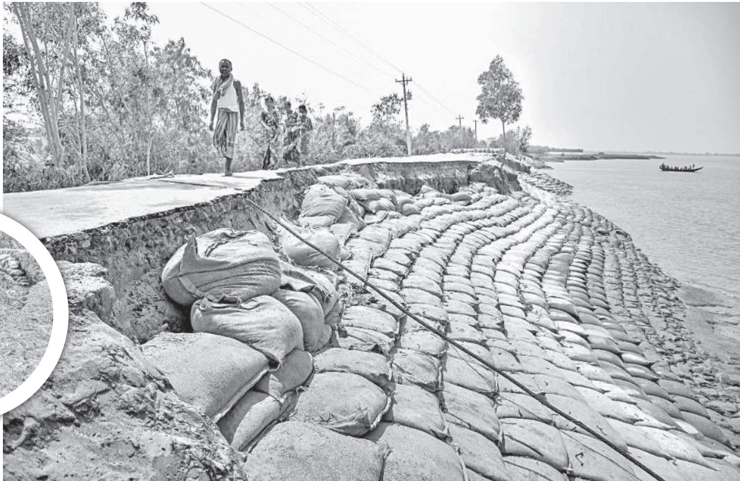
Inhabitants of Sutarkhali and Kamarkhola unions in Khulna's Dacope upazila find themselves gripped by panic as an embankment constructed by the Water Development Board begins to crumble. As the embankment, part of the Coastal Dam Development Project, nears completion; sections, notably in Gunari village of Sutarkhali union, have already been devoured by the river.
