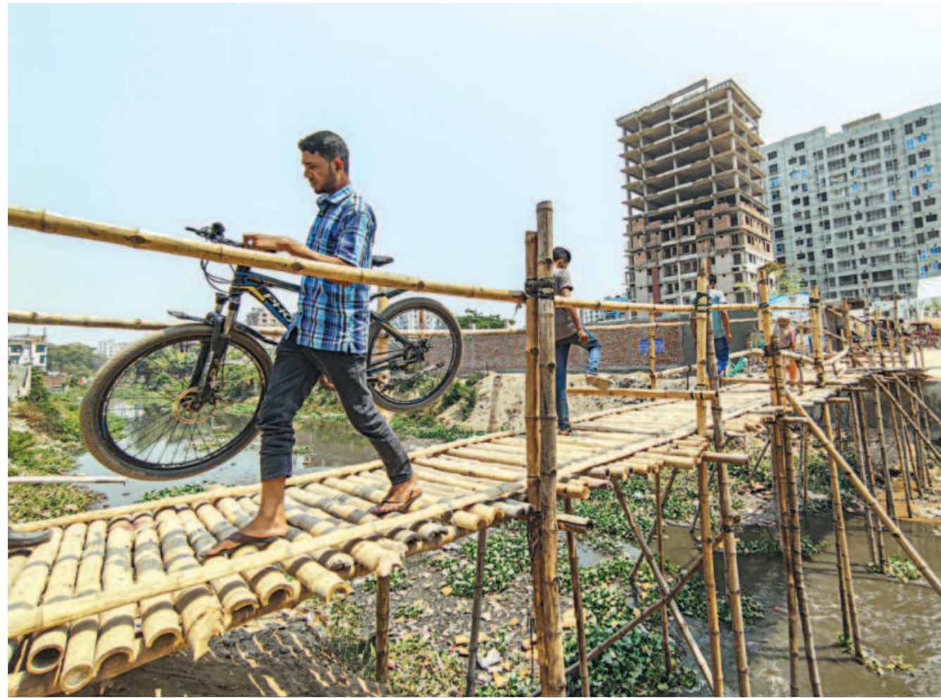
Locals of Bosila and Chandrima Housing in Mohammadpur regularly build such bamboo bridges to cross the Ramchandrapur Canal, located between the two areas. While it is risky for them to cross it, they claimed the authorities concerned have never taken the initiative to build a concrete bridge there.
