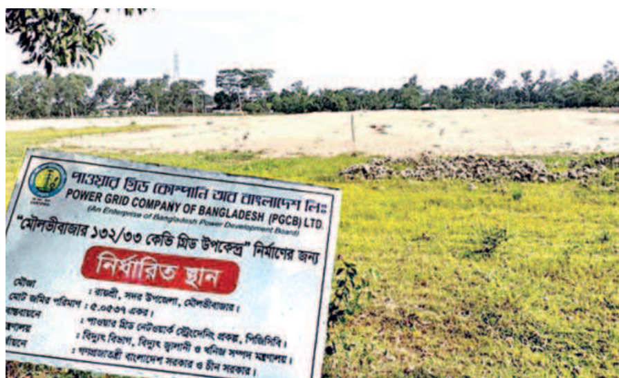
Construction work of Moulvibazar 132/33 KV Grid Substation at Raishree village in Moulvibazar Sadar upazila is going on at a slow pace. PHOTO: STAR
