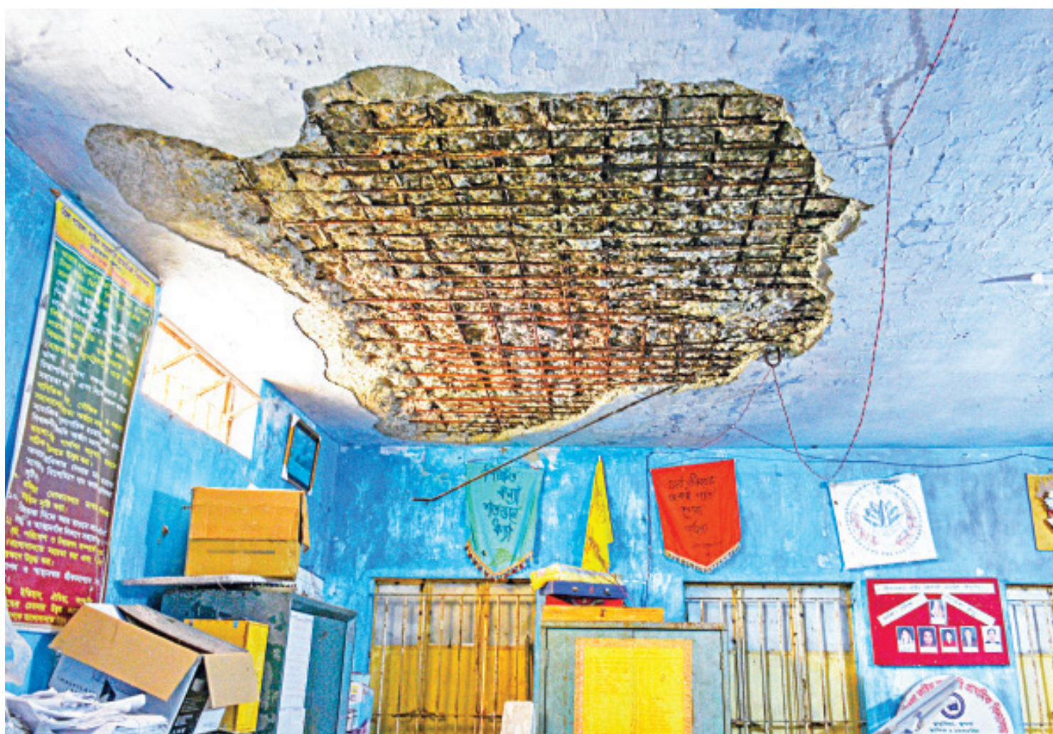
The iron rods of the ceiling can be seen in a room of Bil Pabla Line Government Primary School in Khulna's Dumuria upazila. The two small buildings of the school have not been renovated or restored since they were built in 1996. The loose plaster of the ceiling often falls off putting teachers and students at risk of injuries. The photo was taken yesterday.
