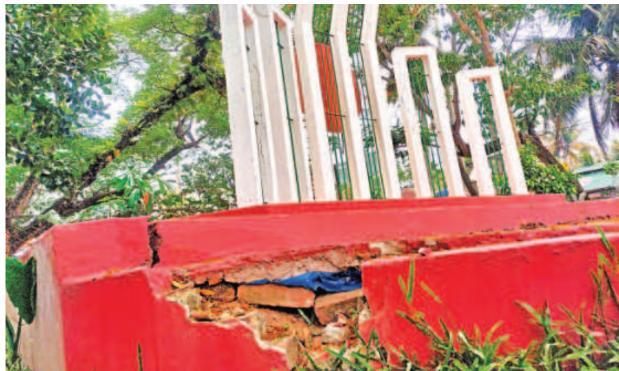
The Central Shaheed Minar in Moulvibazar's Kulaura upazila remains awfully risky, much to the worry of local people. PHOTO: STAR
