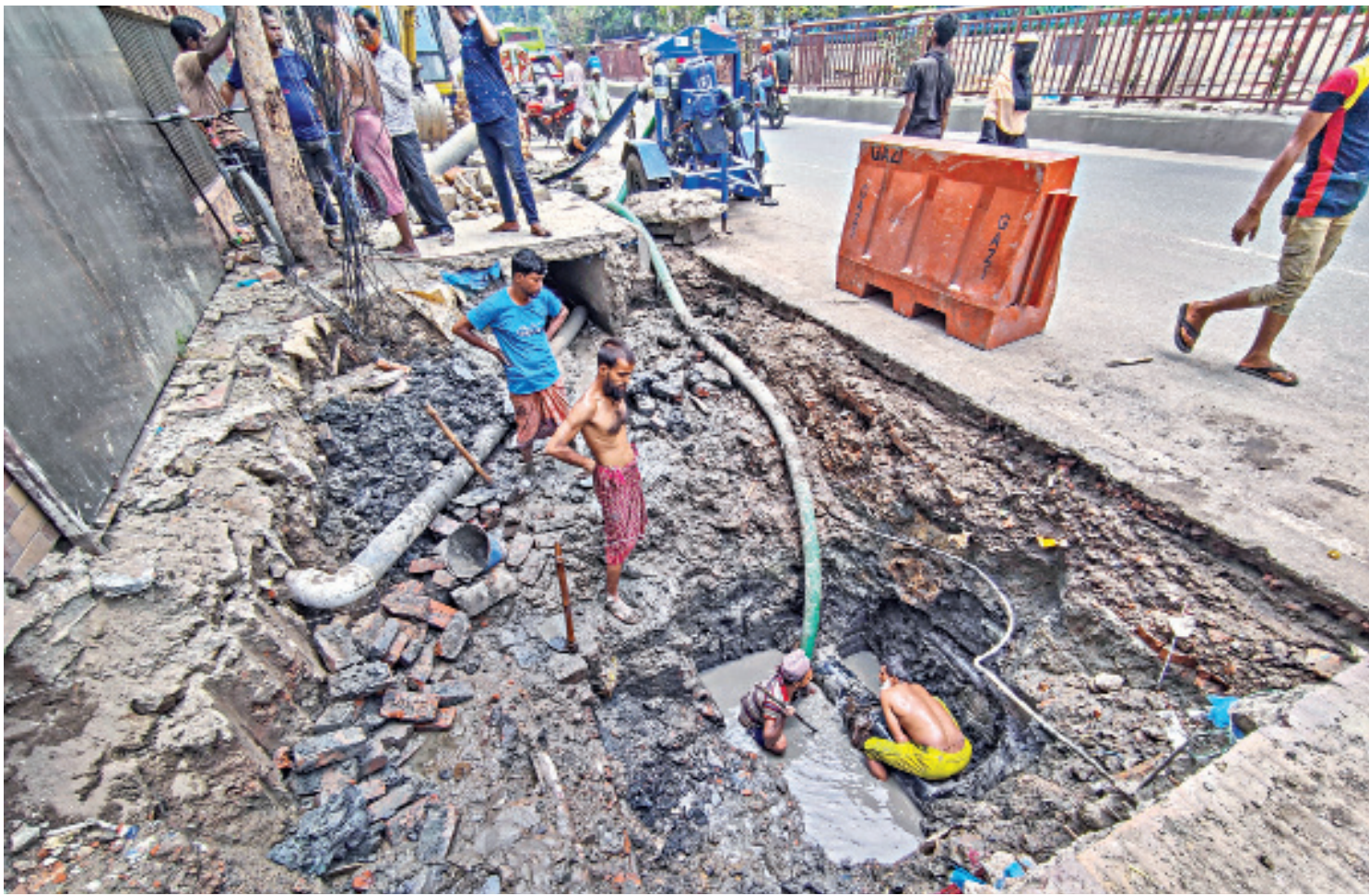
Workers of Dhaka Wasa repairing drainage pipe underneath a footpath on Saat Masjid Road. The pavement has been dug deep, and workers are operating in the drain below without taking any necessary safety precautions. The situation is particularly hazardous at night, as the lack of safety measures increases the risk of someone falling down. This photo was taken in Lalmatia yesterday.
