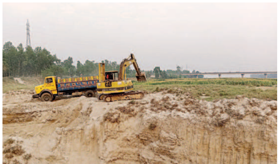
An excavator set by a local syndicate, extracts sand from the Brahmaputra river in Sherpur Sadar upazila, posing threat to the adjacent bridge. PHOTO: STAR
