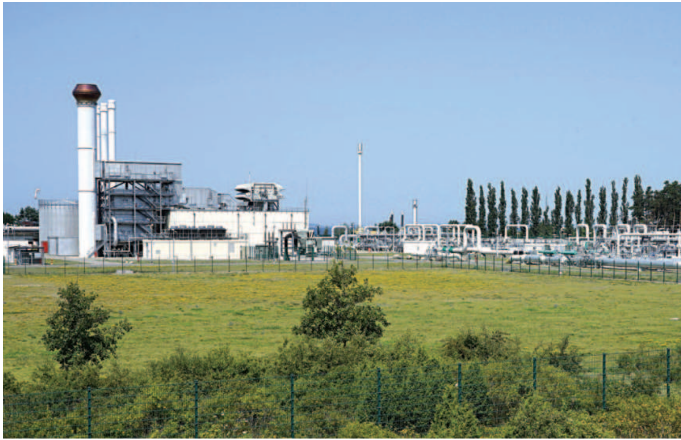
The photo shows pipe systems at the industrial plant of the Nord Stream 1 Baltic Sea pipeline near Lubmin, northeastern Germany. The European and global gas markets suffered a major supply shock in 2022 when Russia reduced its pipeline gas deliveries to the European Union by 80 per cent, triggering a global energy crisis.
