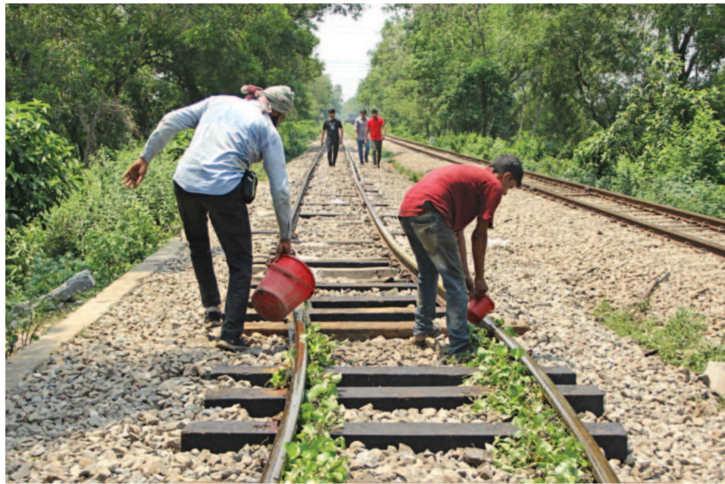
Railway staffers use water and hyacinths to cool down a section of rail tracks which bent due to "excessive heat" in Brahmanbaria's Dariapur area yesterday. Train service between Dhaka and Sylhet and Chattogram was disrupted as only one of the two lines were serviceable.
