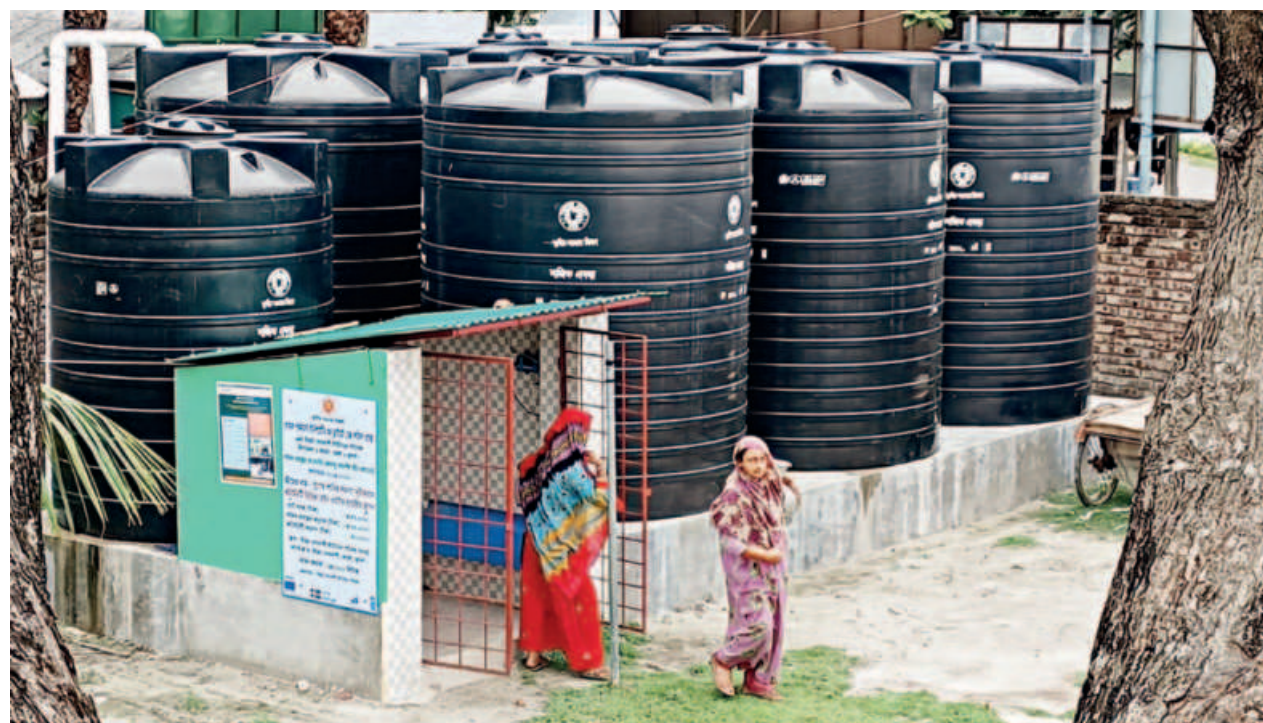
Community women are collecting safe drinking water thanks to rainwater harvesting water treatment plant under PBCRG Scheme
