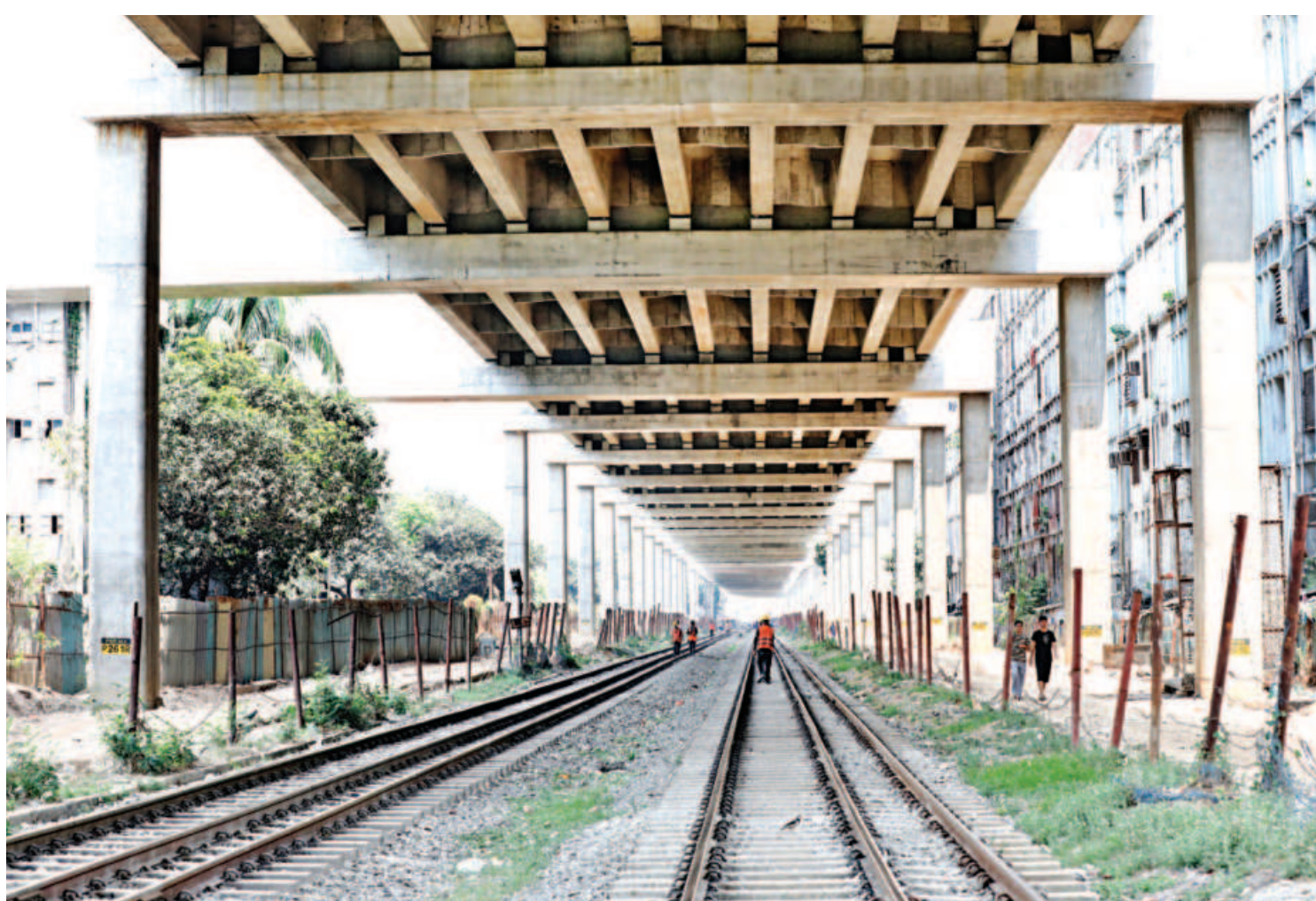
Works of the First Dhaka Elevated Expressway is going on in full swing as the Road Transport and Bridges Minister Obaidul Quader recently announced that construction of the stretch from Dhaka airport to Tejgaon rail gate is expected to be completed by November this year. The 47km expressway, with a 19.73km main line, will run from from HSI A till Kutubkhali. The photo was taken at Chairmanbari in the capital's Banani yesterday.
