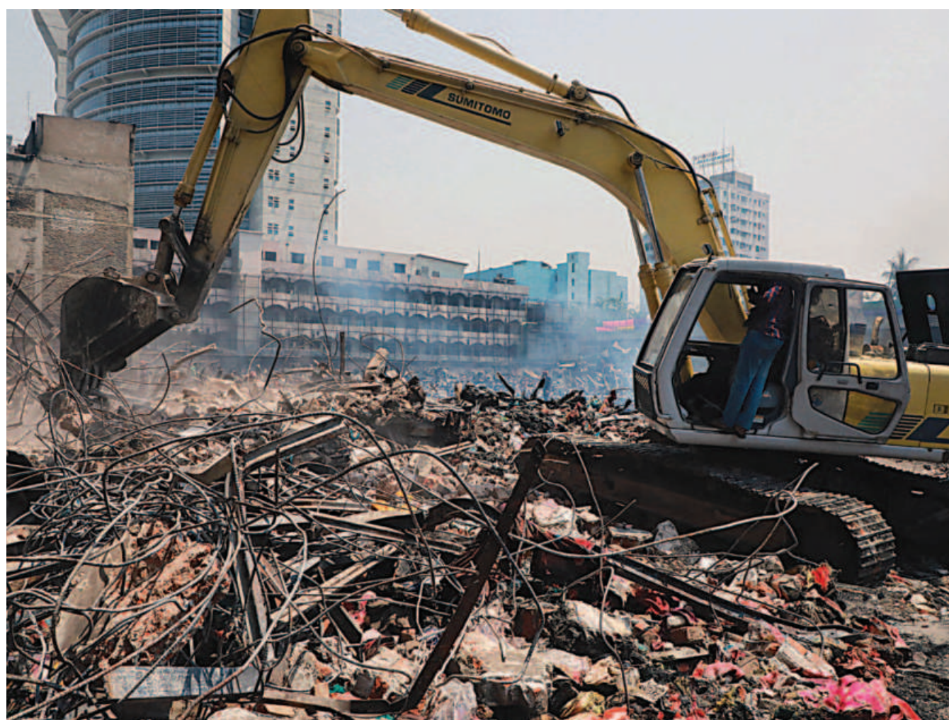
An excavator yesterday removes the debris from Bangabazar, which was destroyed by a massive fire on April 4, as traders are going to start their business on Wednesday by setting up makeshift shops there.
