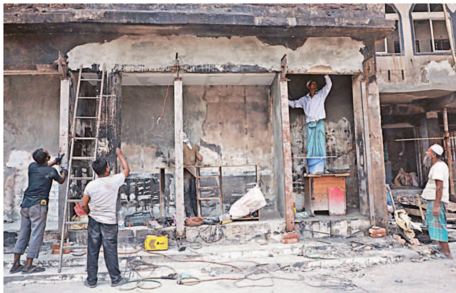
Like other nearby establishments, these shops opposite to Bangabazar shopping complex in Dhaka’s Gulistan area were damaged during a recent fire that broke out at the popular apparel retail hub. Here, workers are seen conducting repairs in hopes of reopening the store before Eid-ul-Fitr. The picture was taken yesterday.
