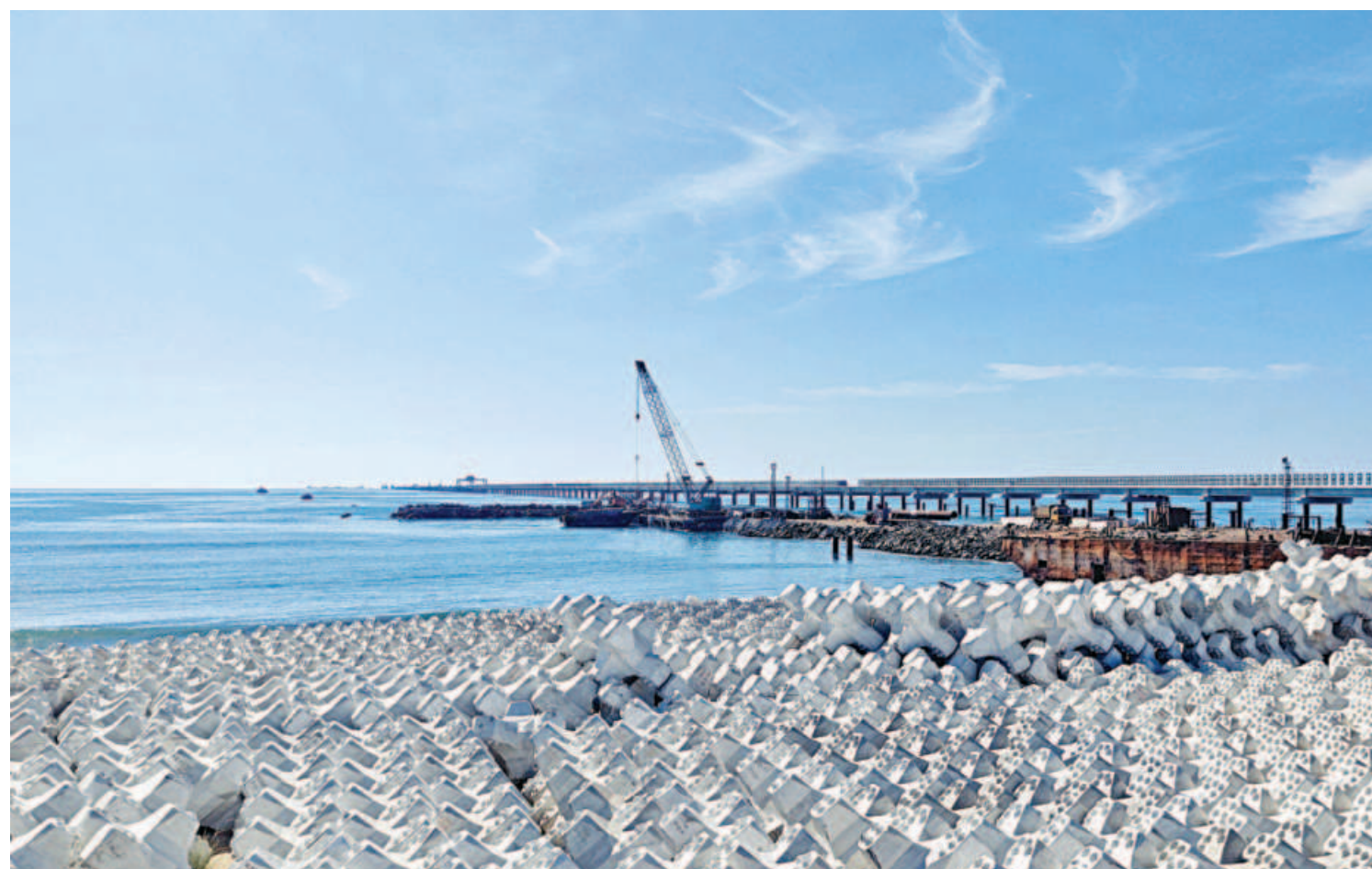
A view of an under-construction coal jetty of a power plant on the coastline near India's southern tip in Udangudi of Tamil Nadu. Intense summer heatwaves, a colder-than-usual winter in northern India and an economic recovery led to a jump in electricity demand, forcing India to crank up output from coal plants and solar farms as it scrambled to avoid power cuts.
