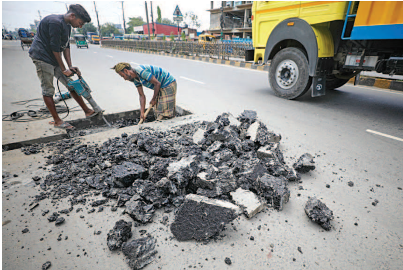
The 6km-long Port Connecting Road in Agrabad being dug up by Chattogram Wasa, just three months after the road was repaired for the smooth plying of vehicles. Locals are blaming both Wasa and the Chattogram City Corporation for this irresponsible move just ahead of Eid-ul-Fitr and the monsoon season.
