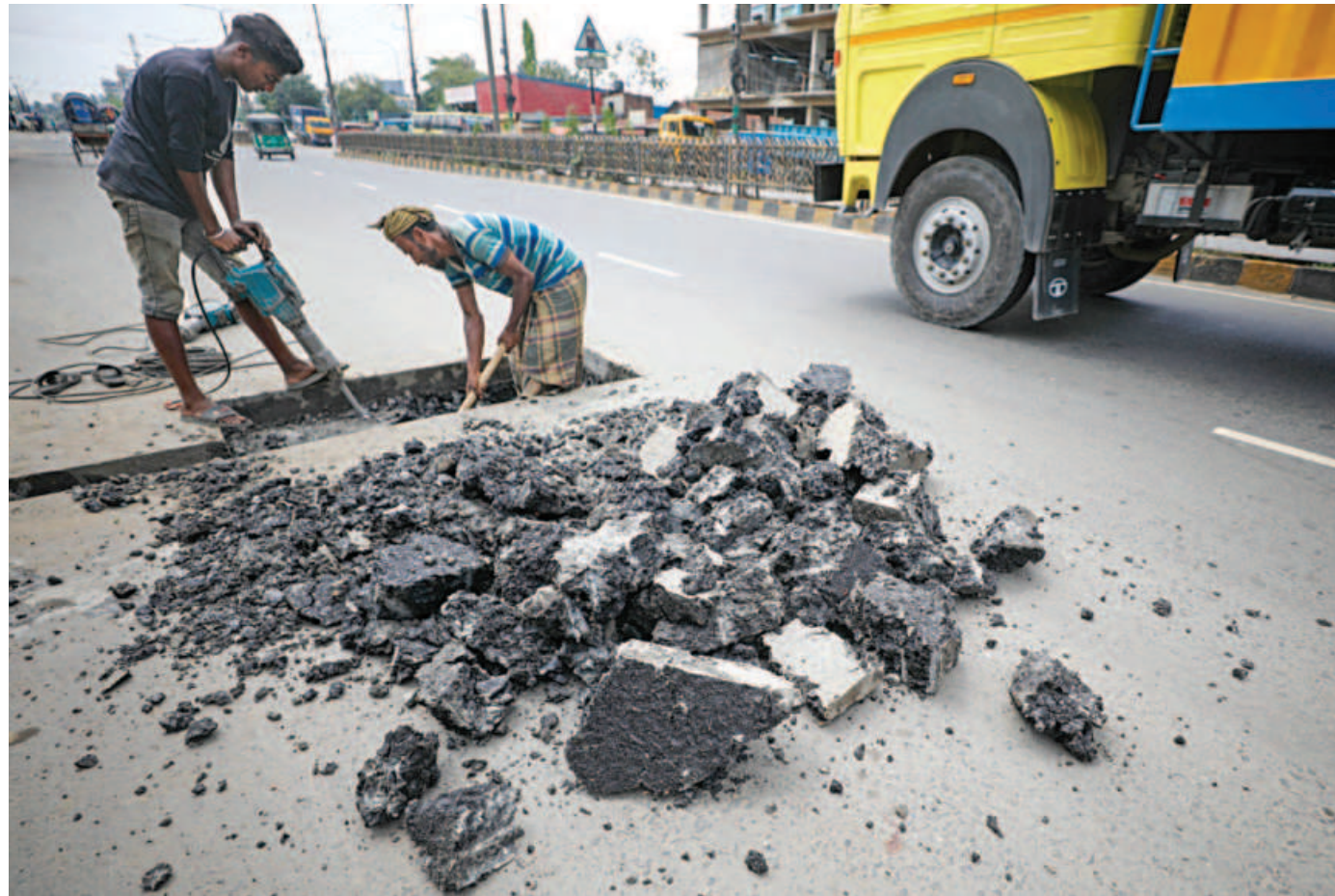
The 6km-long Port Connecting Road in Agrabad being dug up by Chattogram Wasa, just three months after the road was repaired for the smooth plying of vehicles. Locals are blaming both Wasa and the Chattogram City Corporation for this irresponsible move just ahead of Eid-ul-Fitr and the monsoon season.
