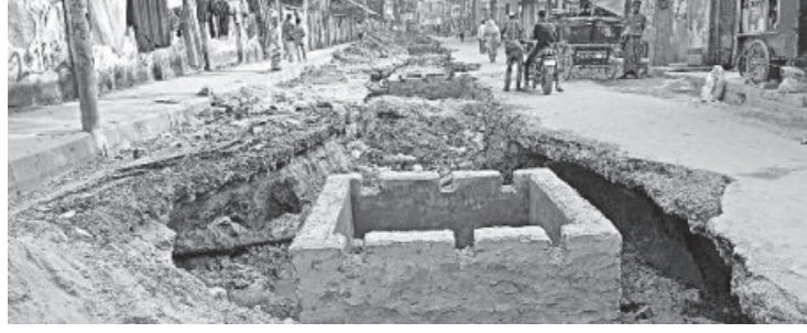
This road has been in this state for around a month now. Due to delay in construction, locals and passersby are having a hard time reaching their destination.
