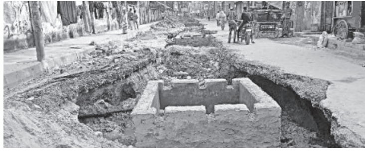
This road has been in this state for around a month now. Due to delay in construction, locals and passersby are having a hard time reaching their destination.
