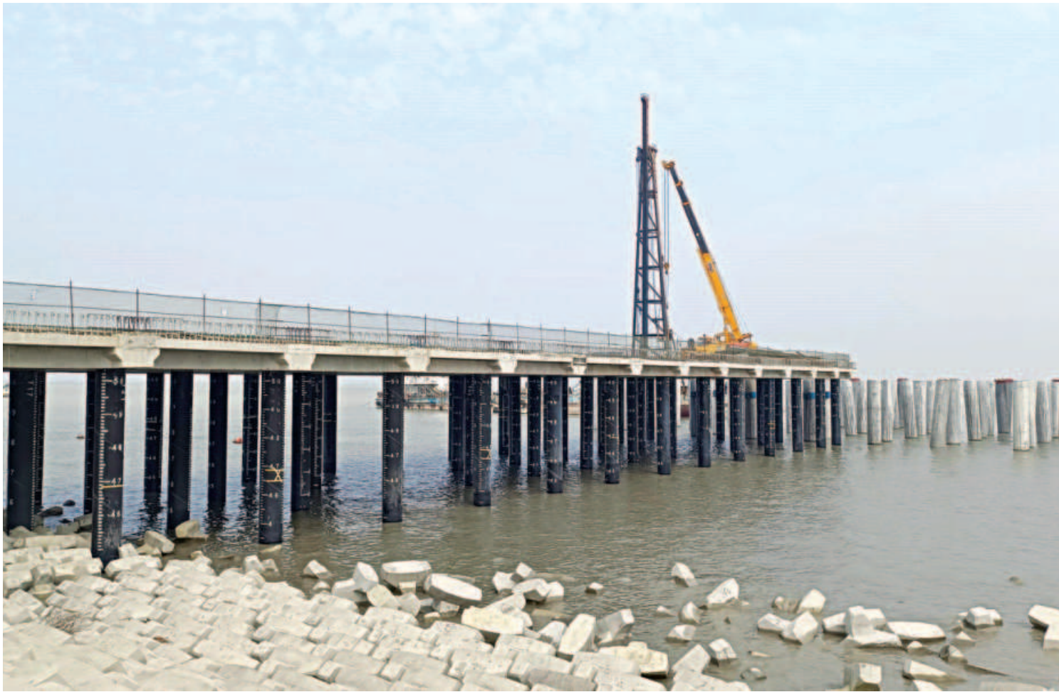
As construction of the first terminal of Payra Port nears completion, larger vessels are expected to arrive as early as the first week of April. While the largest ship to berth at Chattogram port had a draft of 9.50 metres, vessels with a draft of 10.5 metres will be able to sail into Payra port once the project ends.
