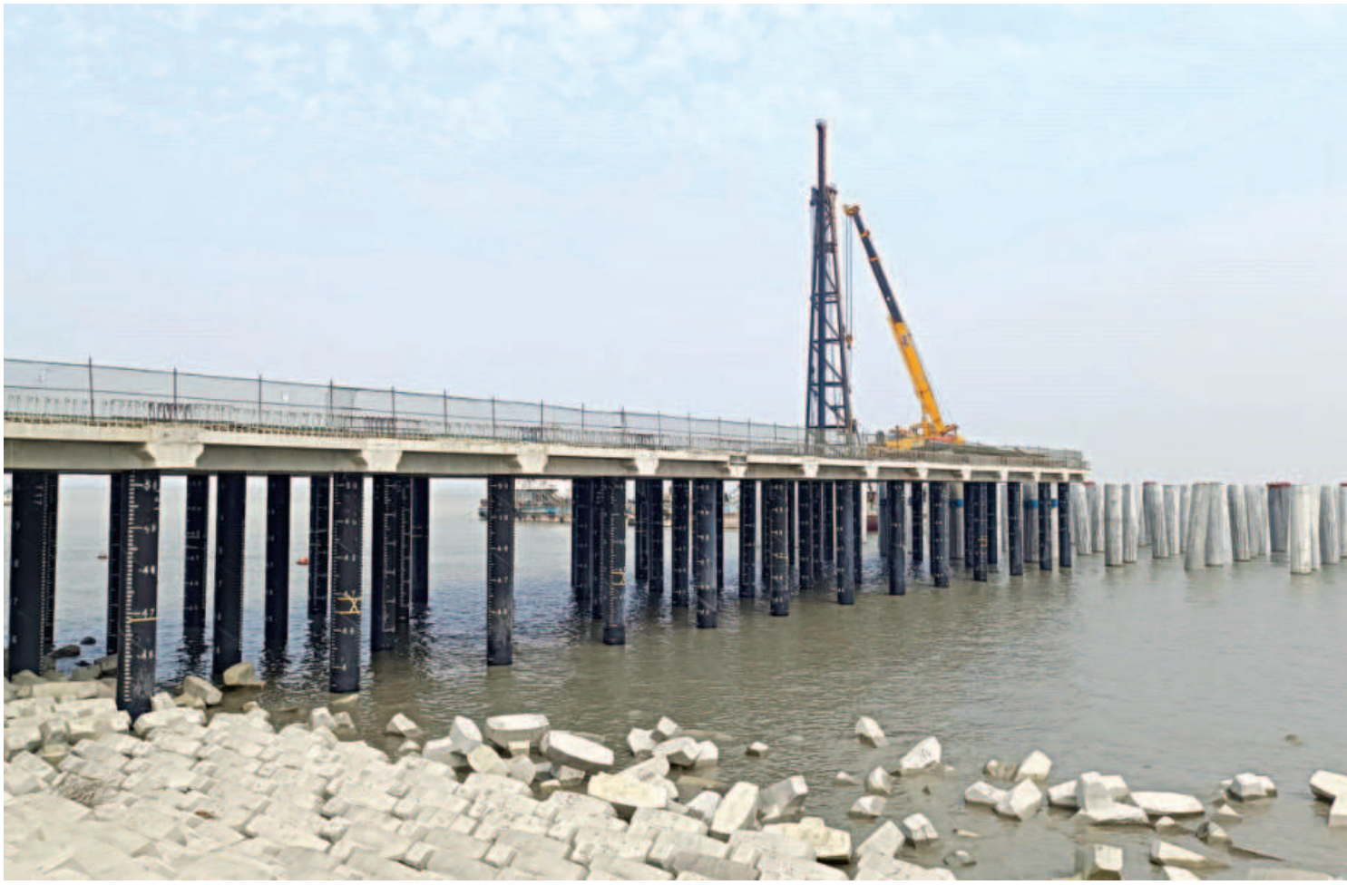
As construction of the first terminal of Payra Port nears completion, larger vessels are expected to arrive as early as the first week of April. While the largest ship to berth at Chattogram port had a draft of 9.50 metres, vessels with a draft of 10.5 metres will be able to sail into Payra port once the project ends.
