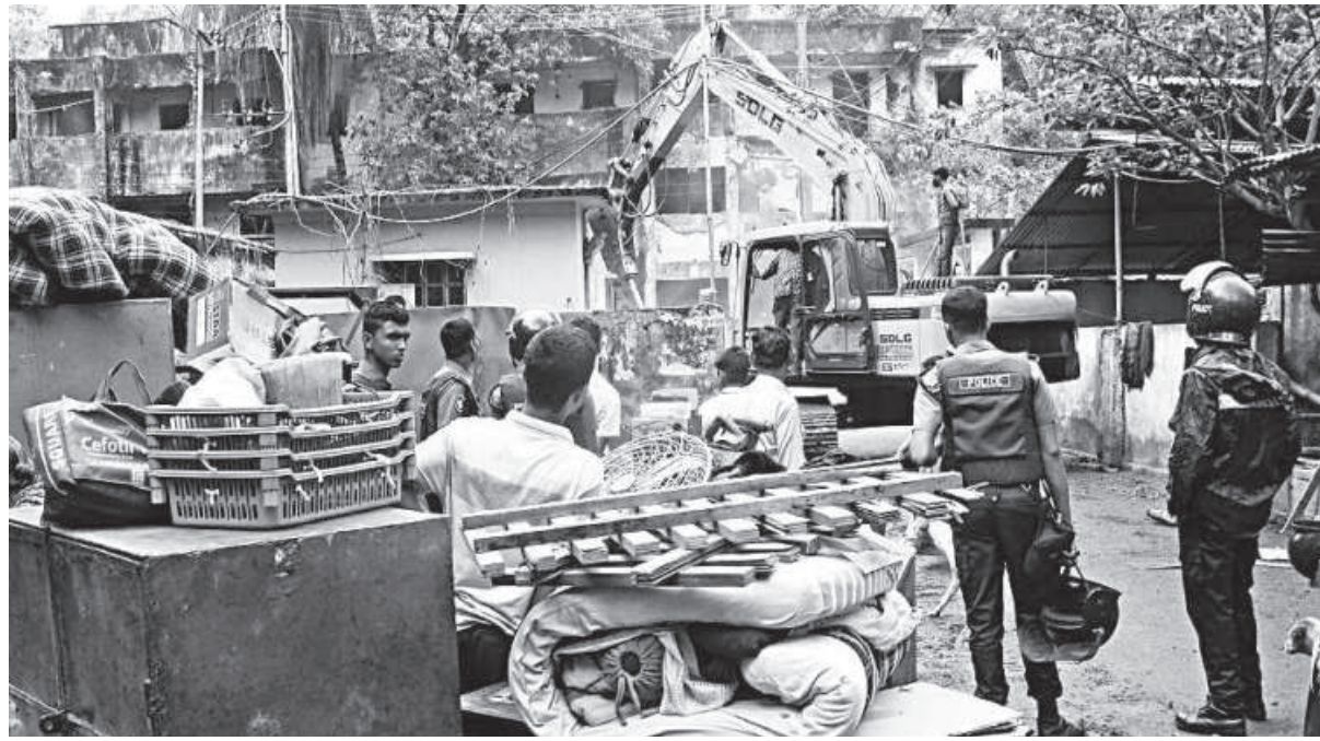
A mobile court of Chattogram District Administration yesterday demolished more than 300 illegal structures built on Chattogram Medical College Hospital land. The authorities conducted the drive to pave the way for a multi-storey 150-bed modern burn and plastic surgery unit. PHOTO: STAR
