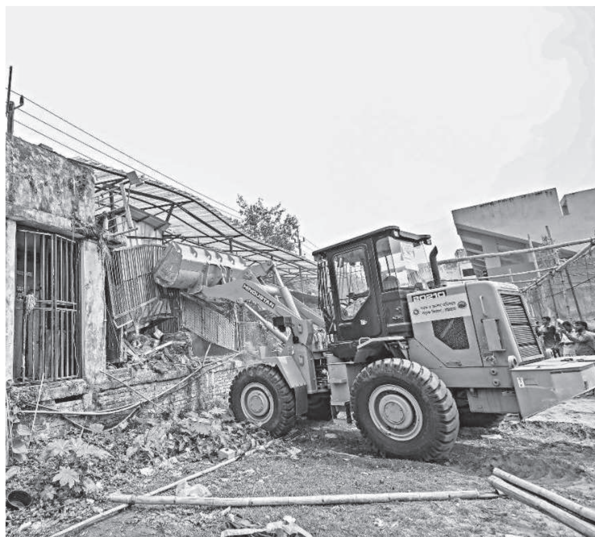
Chattogram District Administration demolished 15 establishments -- including two restaurants -- in the city's Outer Stadium area yesterday to recover the playground.
