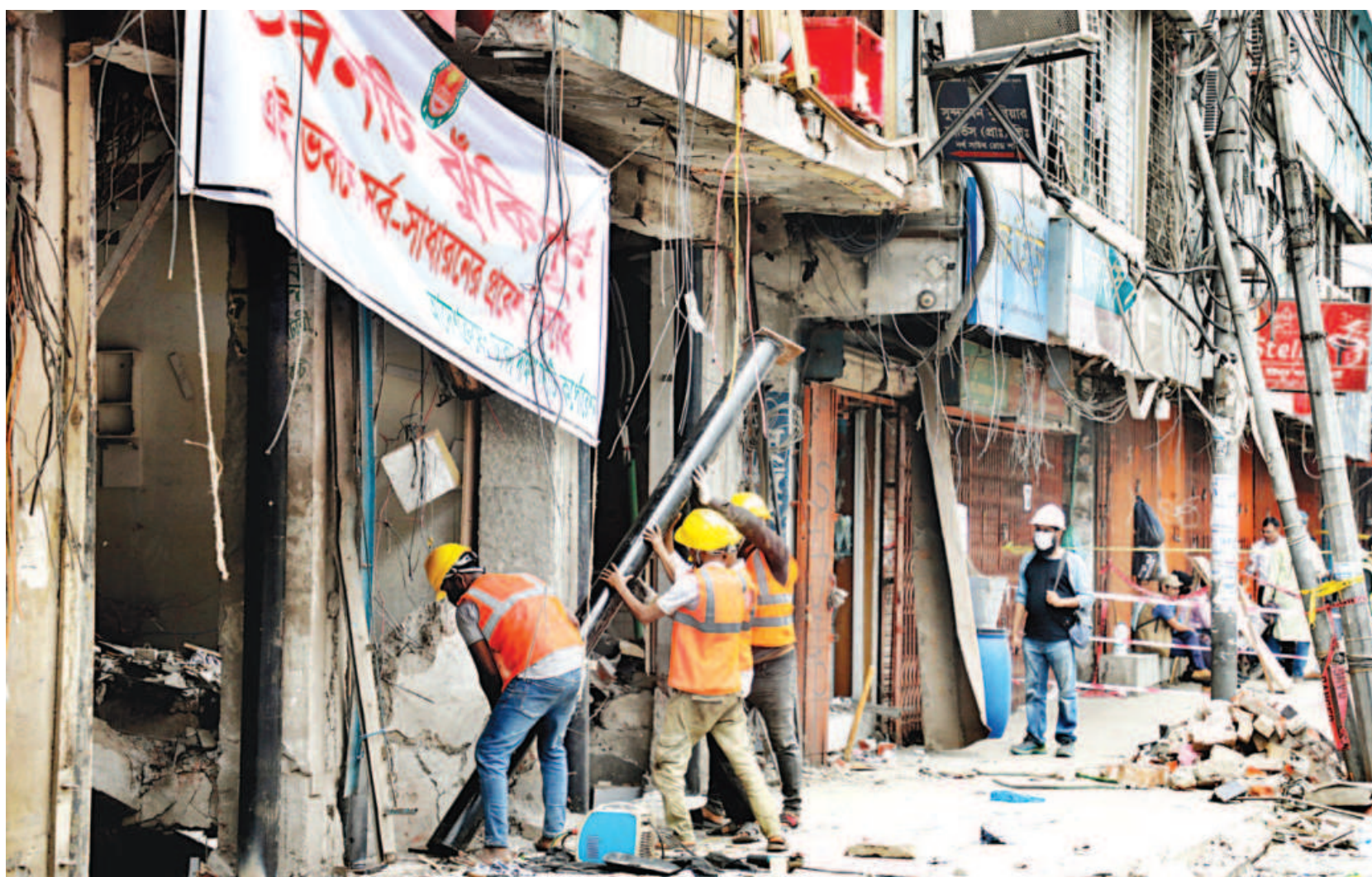
Workers moving an iron pole to prop up a beam of the seven-storey building on North South Road in the capital's Siddikbazar yesterday. A massive blast at the building on Tuesday killed at least 22 people and injured over 100 others.
