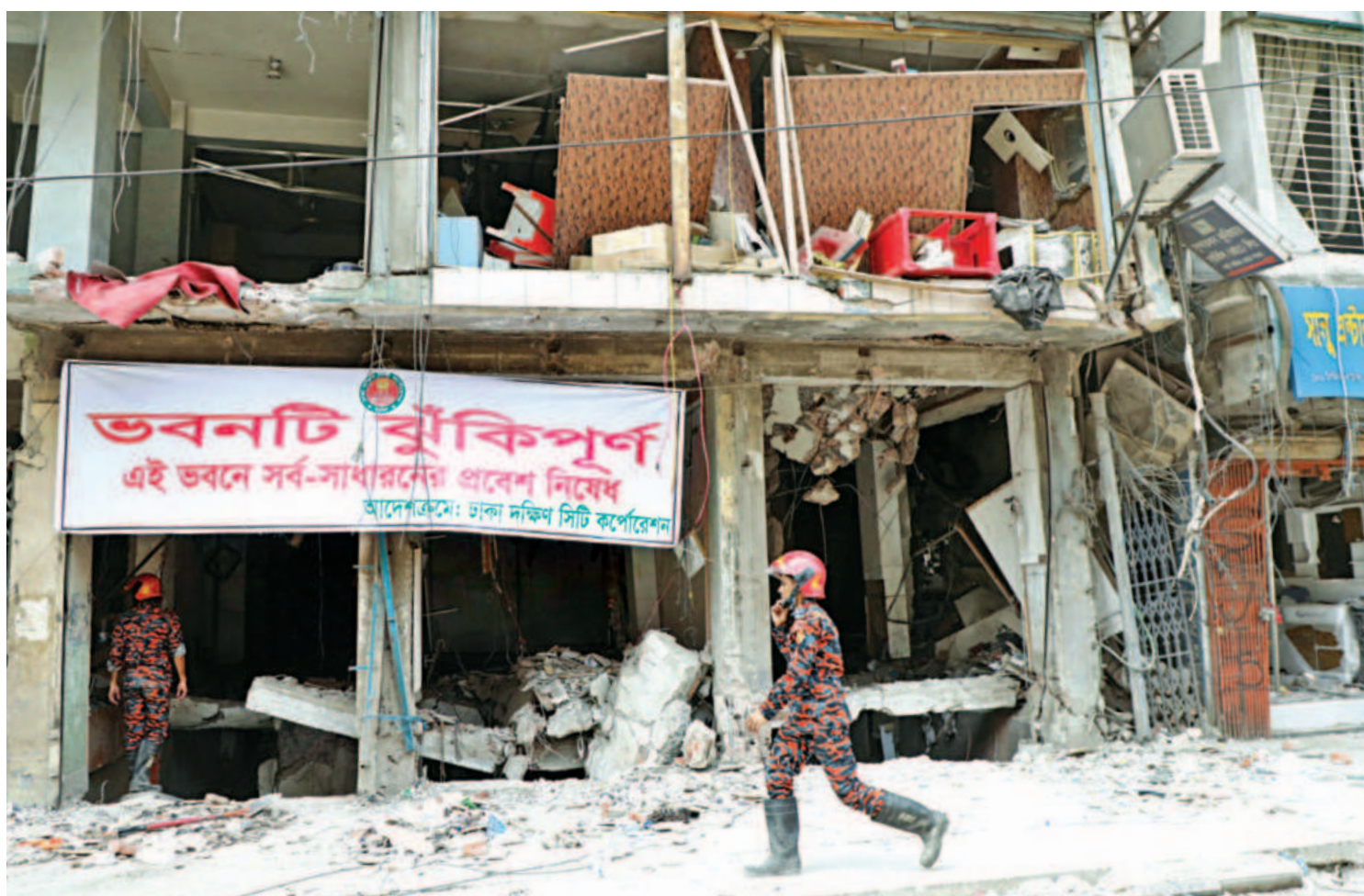
Two rescuers at the scene of an explosion at the seven-storey building on North South Road yesterday. Dhaka South City Corporation has put up a banner on the structure declaring it risky and prohibiting people from entering it. The blast on Tuesday left at least 22 people dead and over 100 others injured.
