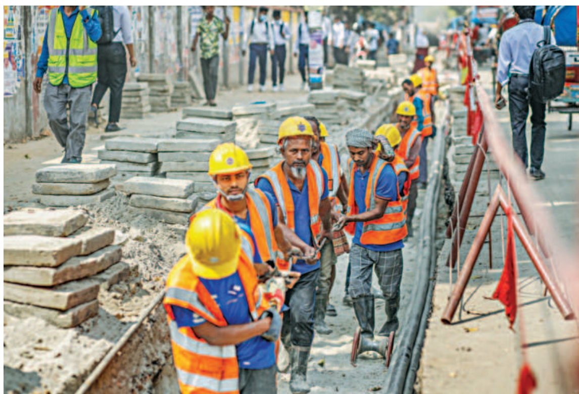
Workers installing underground cables on Satmasjid Road in Lalmatia yesterday. Dhaka Power Distribution Company (DPDC) is conducting the work.
