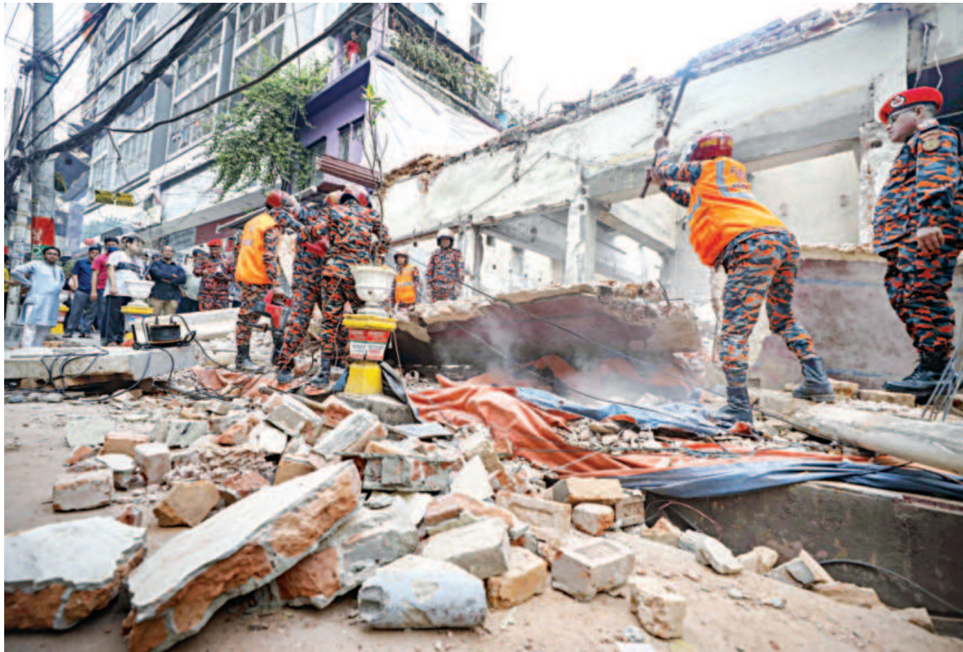
Firefighters clear rubbles from a pavement in Chattogram city's Jamal Khan area yesterday afternoon after a wall of a building collapsed during its demolition. The incident left a demolition worker dead and another man injured.
