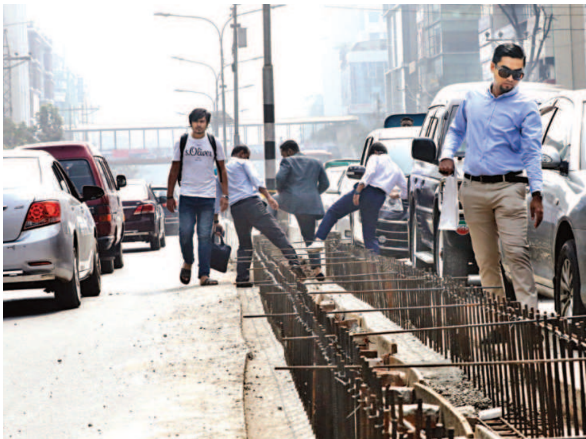
A footbridge is not far, but people are choosing to walk through the obstacles of the under-construction road divider to go across Sat Masjid Road in the capital. Besides, the risk of getting pierced by the pointy rods, they also risk being runover by vehicles.
