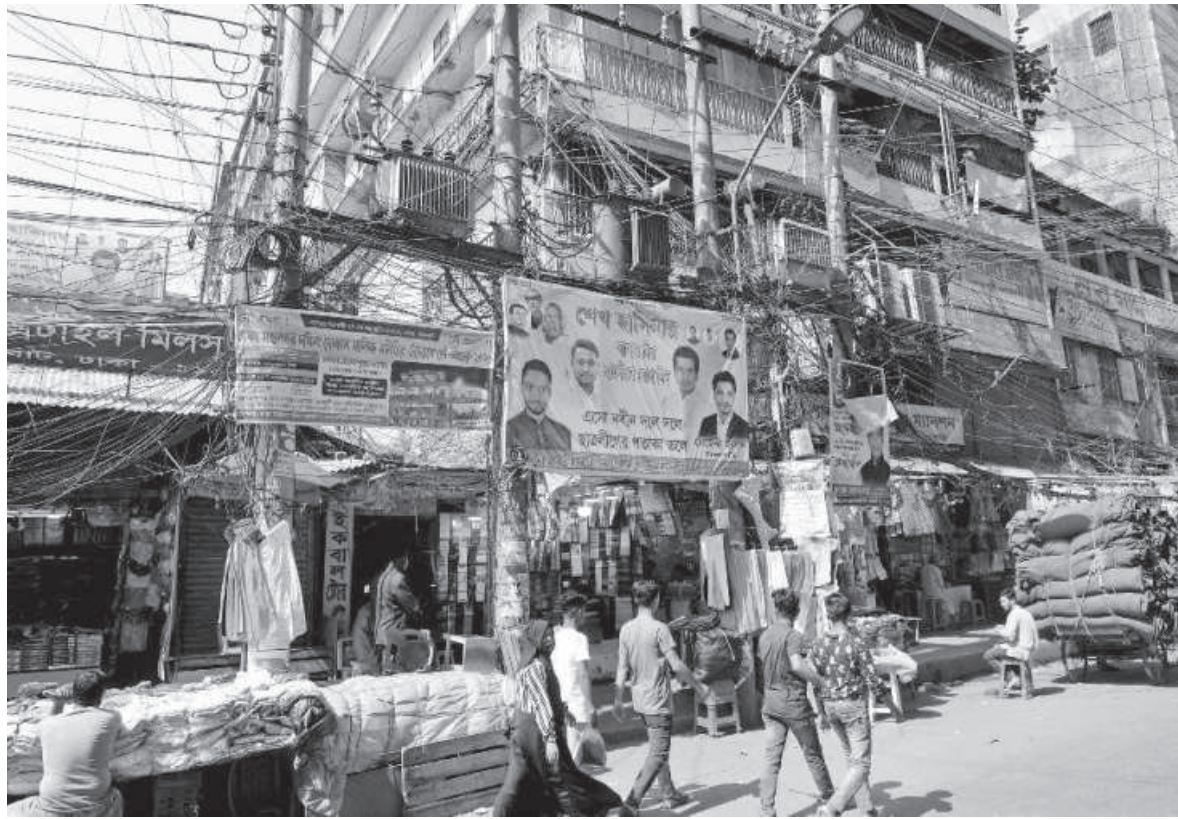
Jumbled electric wires hang from an electric pole overhead, while vendors sell clothes right beneath them, unaware of their safety. At any point, if the sparks of the wire get caught in the clothes, a grave accident may occur. This photo was taken in Chittaranjan Avenue of the capital's Sadarghat yesterday. PHOTO: PALASH KHAN
