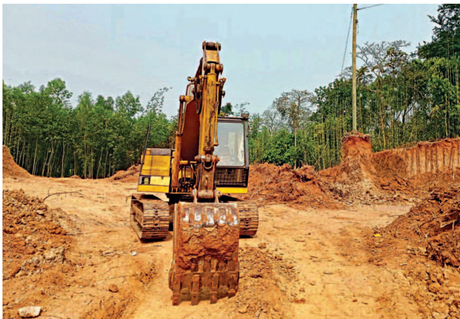
Soil traders are razing hillocks in Tarafpur of Tangail's Mirzapur upazila, putting the environment at risk. The earth extracted from the hillocks would be used for making bricks, filling low land and building roads. The photo was taken recently. Story on page 5. PHOTO: STAR
