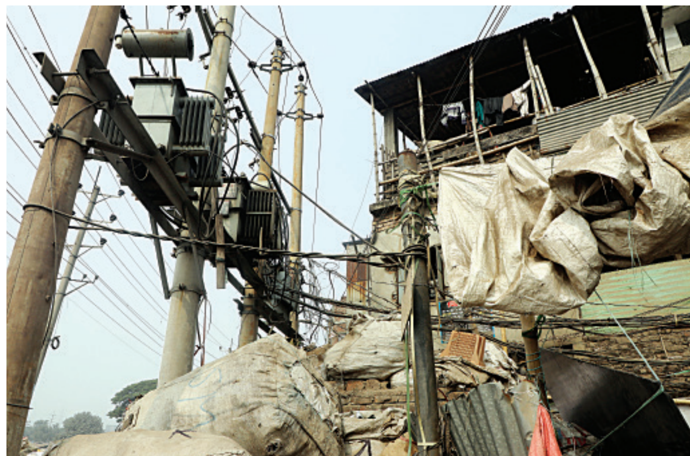
Traders have stacked large bags full of discarded plastic bottles right under electricity transformers at Islambagh in the capital's Lalbagh, putting the area at risk of fire. Some of the bags are in direct contact with electricity cables connected to the transformers. The photo was taken recently.
