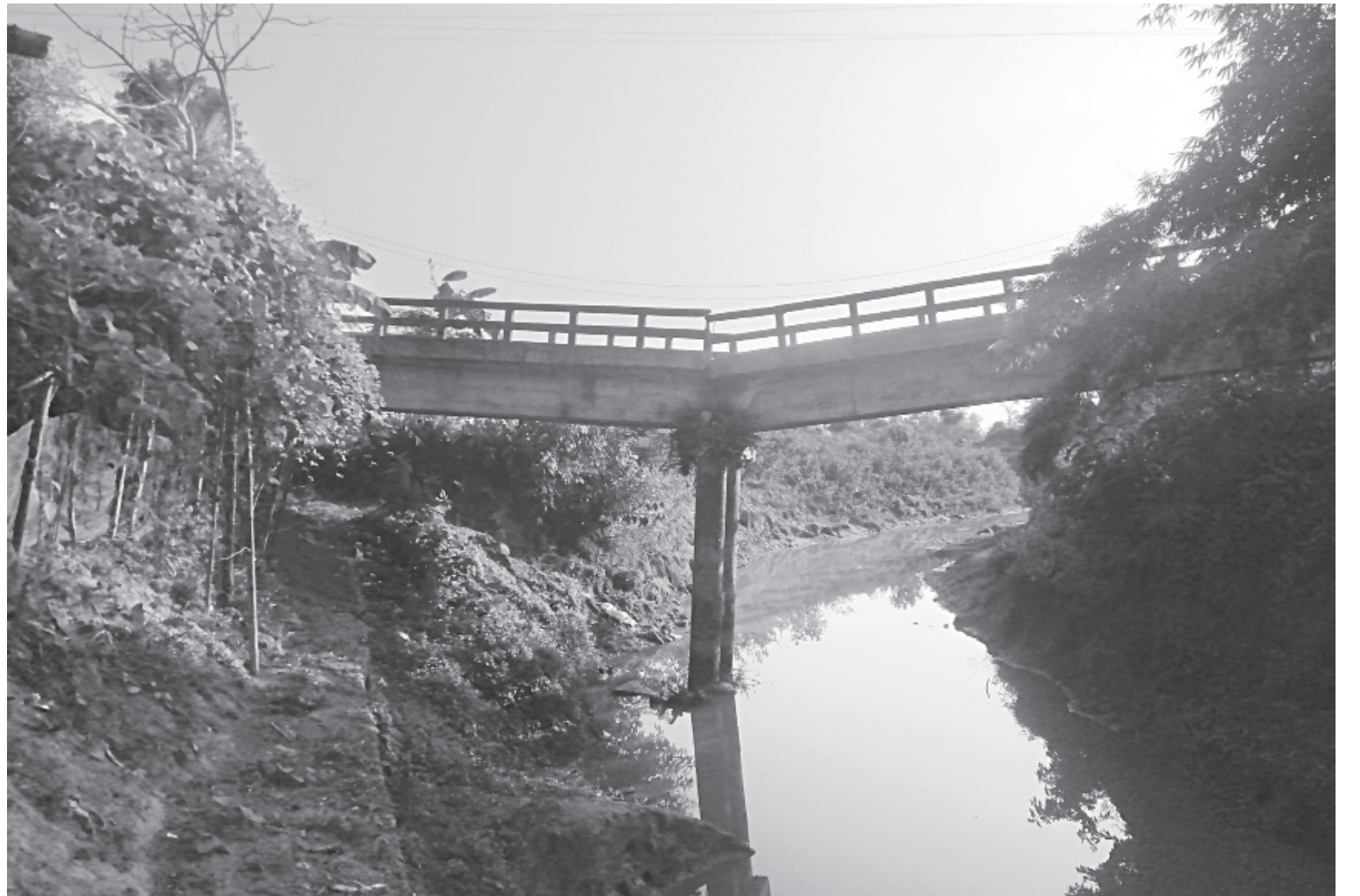
This bridge on Hashimpur-Laxmipur road in Moulvibazar's Kulaura upazila has partially collapsed due to alleged unplanned dredging of the Fanai river.
