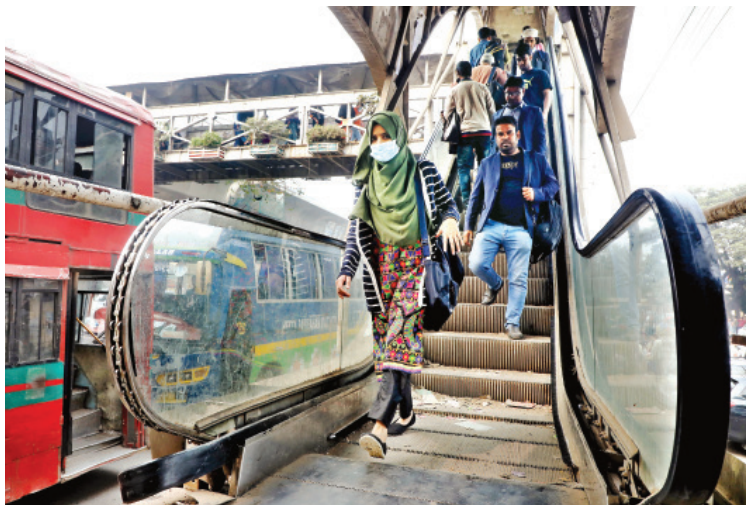
The escalator-equipped footbridge in front of the Dhaka airport used to be a relief for pedestrians, especially the elderly and the ones carrying heavy bags. However, the escalator broke almost two months ago and people now climb up and down the staircase.
