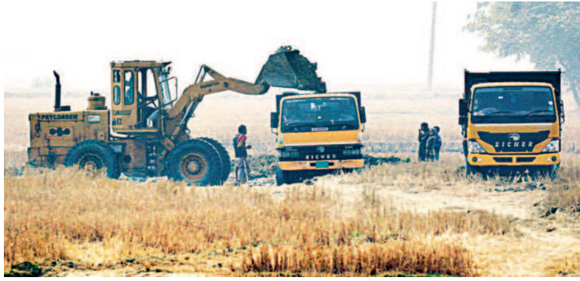
An excavator scoops topsoil from arable land and loads it onto a truck likely bound for a brick kiln. Despite it being illegal, the lack of law enforcement oversight allows influential people to intimidate farmers into selling the fertile layer of the soil, jeopardising future crop yield. The photo was taken yesterday in Gachhbari area of Sylhet's Kanighat upazila.
