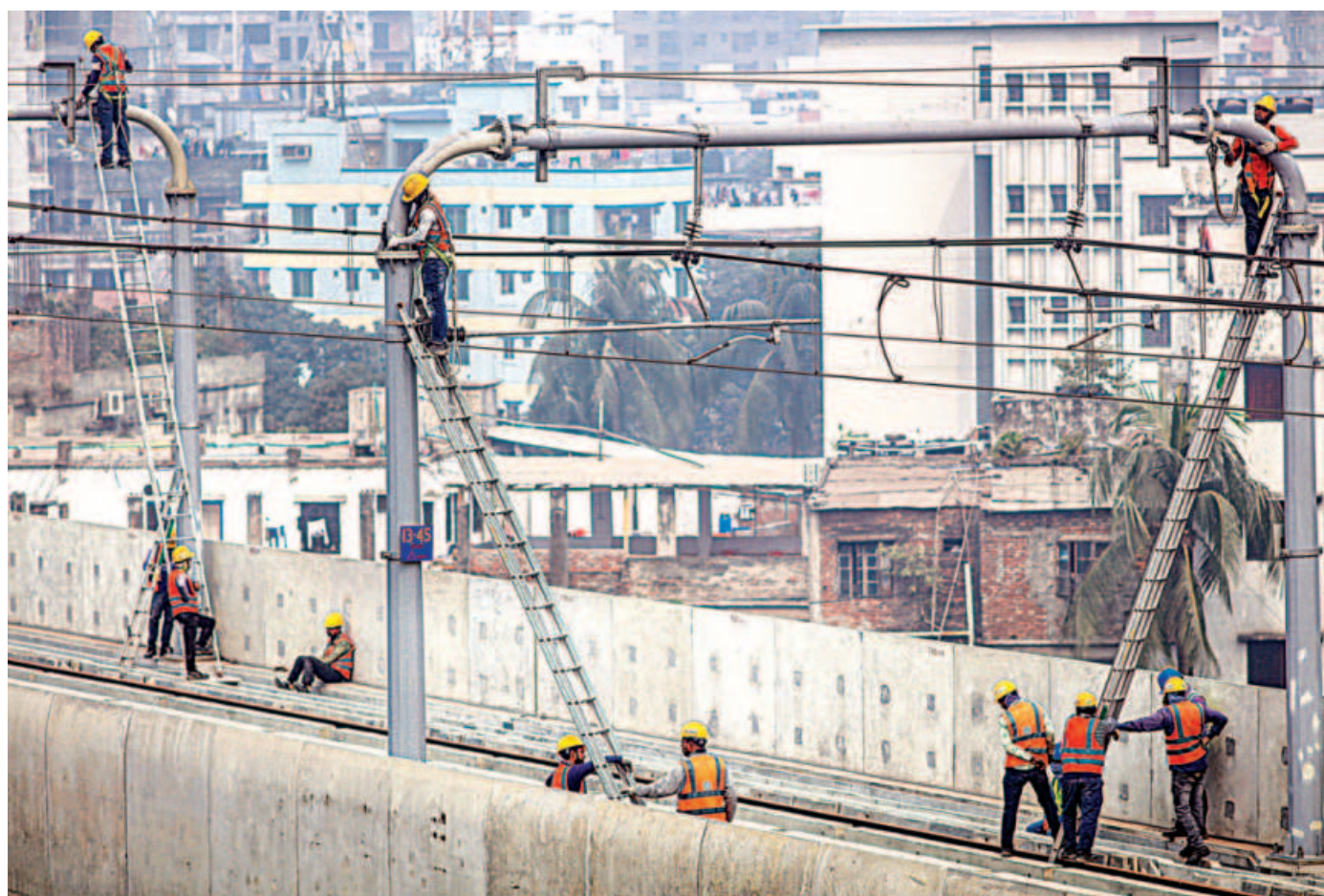
Workers installing power cables and other equipments on the Agargaon-Motijheel section of the metro rail line in the capital's Farmgate yesterday. This segment of the MRT Line-6 is scheduled to be opened to public by this December. PHOTO: RASHED SHUMON
