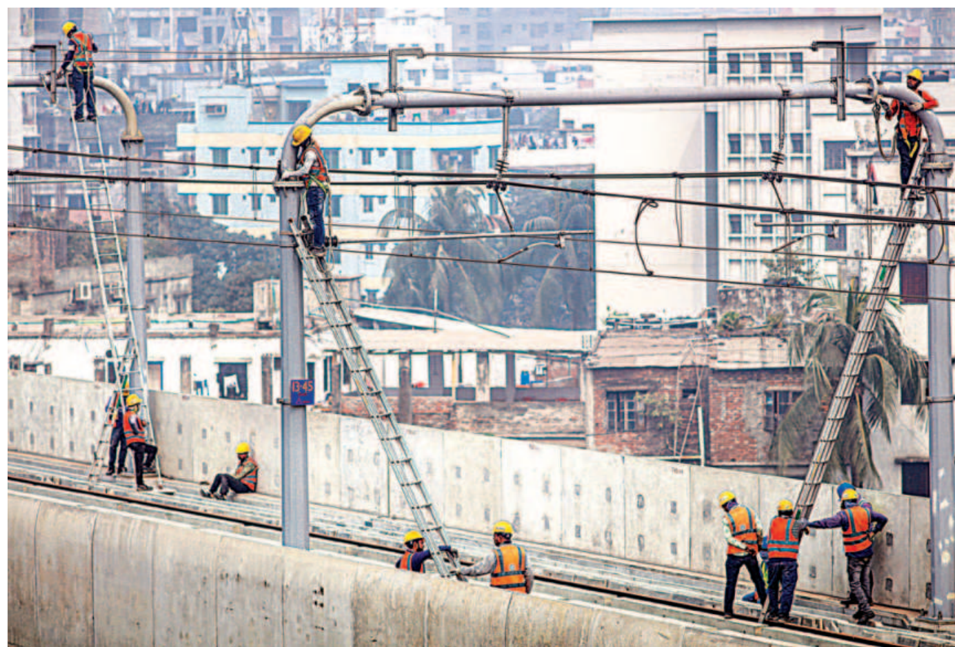
Workers installing power cables and other equipments on the Agargaon-Motijheel section of the metro rail line in the capital's Farmgate yesterday. This segment of the MRT Line-6 is scheduled to be opened to public by this December.
