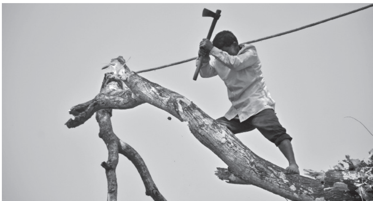
In order to widen Dhaka-Barishal highway, the authorities have decided to cut trees on the side of the road. Although there's a rope to ensure that the branch doesn't fall on the road and injure passers-by, there's no harness to save the man cutting the branch from a deadly fall. This photo was taken recently.
