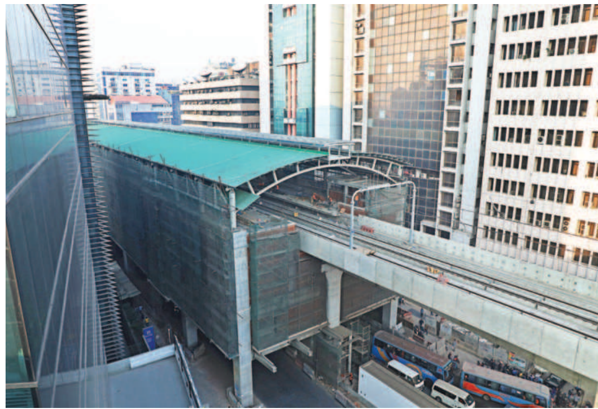
Abdul Monem Ltd, one of the leading infrastructure developers in Bangladesh, constructed the Dhaka metro rail's 3.2km viaduct and three stations from Agargaon to Karwan Bazar under joint ventures with foreign companies. The government launched the country's first metro rail partially on December 28.
