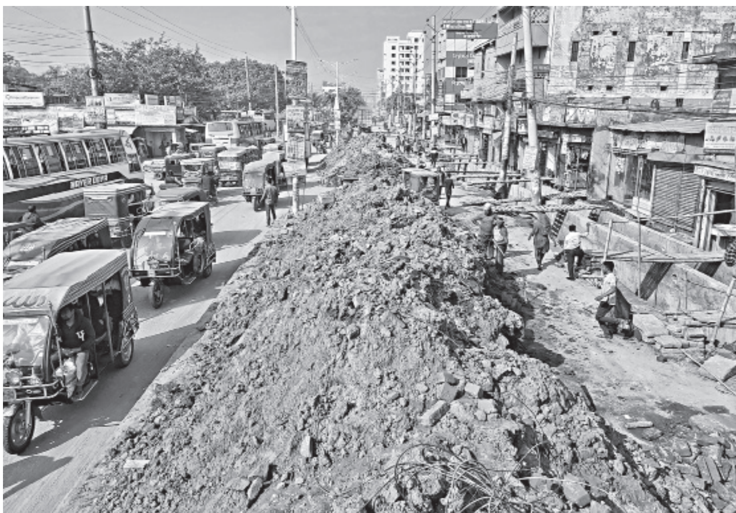
As the city's drainage renovation under Khulna City Corporation goes on in slow pace, commuters suffer long hours on the road, waiting in traffic. This photo was taken in front of Khulna's Sonadanga Bus Terminal yesterday afternoon. PHOTO: HABIBUR RAHMAN
