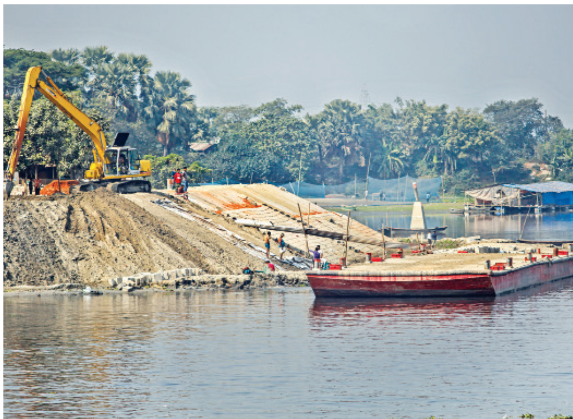
In an attempt to stop river erosion and encroachment, BIWTA authorities have taken up the initiative to set up concrete blocks on the bank of Turag river near Mirpur's Diabari. This photo was taken recently.
