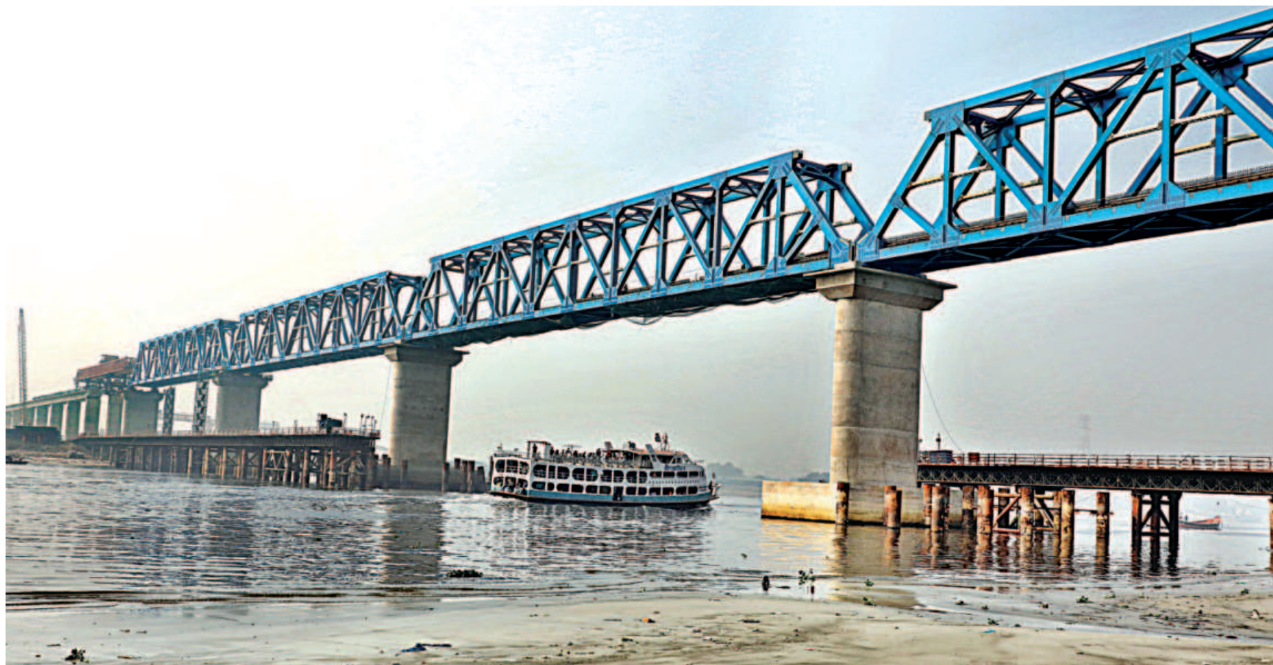
The first railway bridge over the Buriganga is being constructed in Aliganj area of Narayanganj. The rail line will connect the capital with Padma Bridge and the authorities are aiming to operate trains on it by next June.
