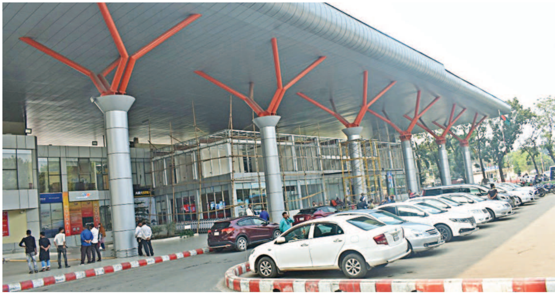
Development works are currently underway at the Saidpur airport in Nilphamari to ready the facility for international flights. With construction of a new terminal almost complete, the airport will soon be able to handle up to 610 passengers at a time. The picture was taken recently. PHOTO: EAM ASADUZZAMAN
