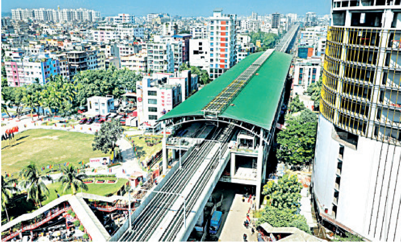
Construction work of the metro rail near the Mirpur-10 intersection. The photo was taken in January, 2022.
