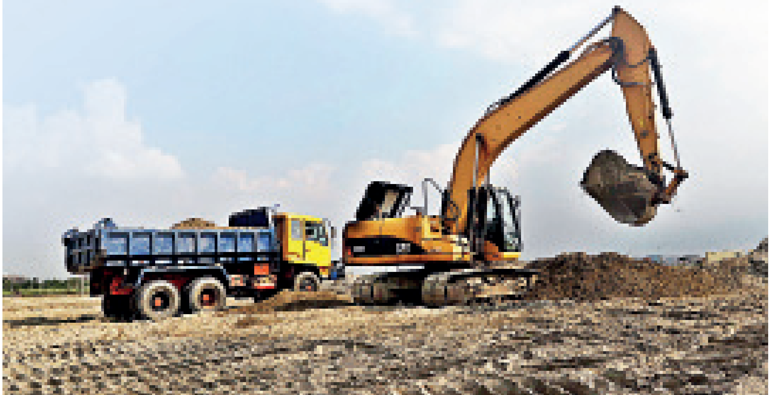
An excavator at a metro rail depot site at Dia Bari of Uttara where the construction work of the country's first metro rail service began on June 26, 2016.
