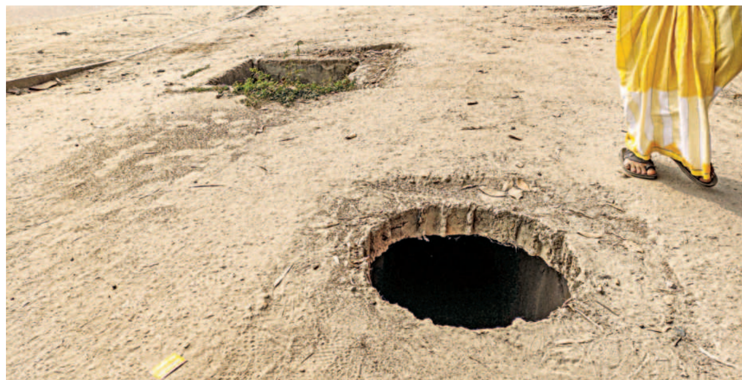
There are several lidless manholes on the entire stretch of the road from Agargaon Shishu Mela to Sher-e-Bangla Nagar area. Several pedestrians have injured themselves by falling into these holes in the last few months, locals claimed. The risks get worse during the night. This photo was taken from Agargaon yesterday.
