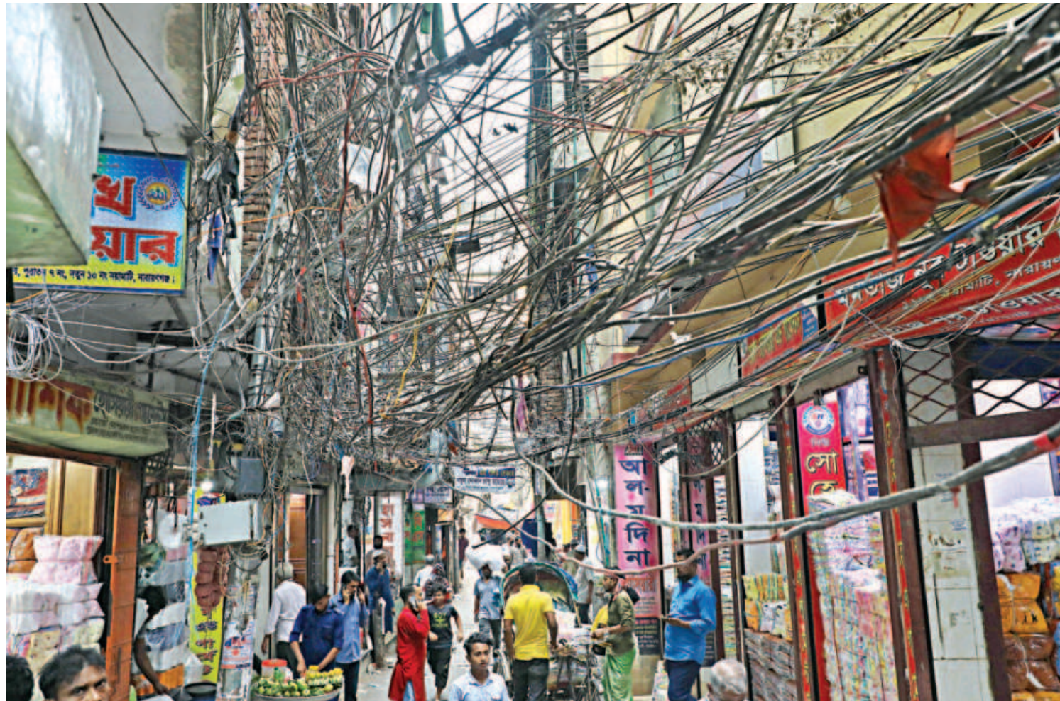
The ugly, tangled mess of overhead cables in Narayanganj's Nayamati area not only blemishes the skyline but also exposes pedestrians to great risks of accidents. The already concerning situation is exacerbated by the fact that this road is always full of people, as shops are situated on both sides. This photo was taken recently.
