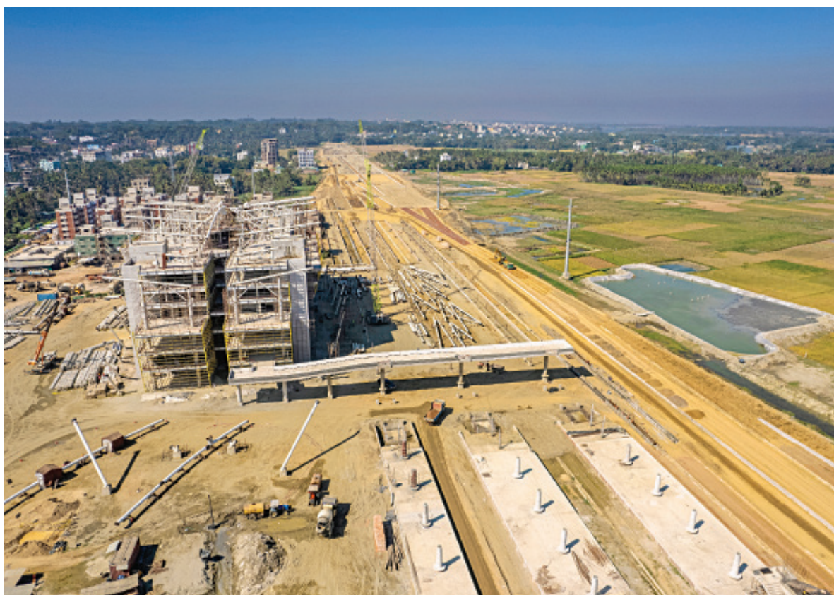
The construction of an iconic railway station in Ramu upazila of Cox's Bazar has been going on in full swing. Once built, the oyster-shaped station on 29 acres of land will connect the district with Chattogram and the rest of the country. The photo was taken in Ramu's Chandherpara area recently. PHOTO: RASHED SHUMON
